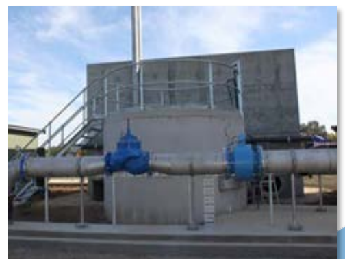
RIGHT: MEDIA FILTER TANK, FILTER WATER TANK AND BACKWASH INLET PIPELINE
